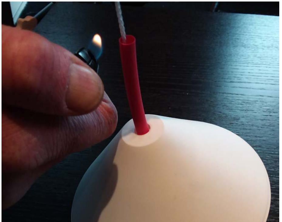
Figure 9: Step 8 - Use firelighter to shrink the upper third of the tube so that rainwater cannot easily enter the rigid tube.
